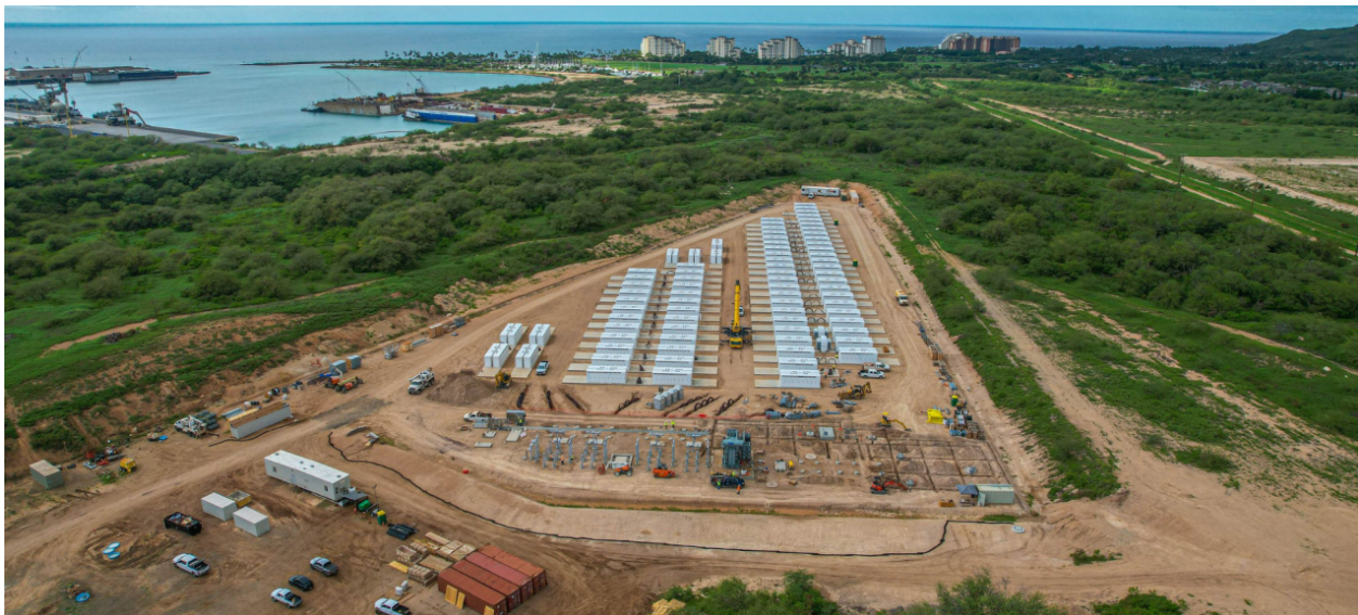
Construction at the Kapolei Energy Storage Facility on Oahu. Source: Goodfellow Bros.
